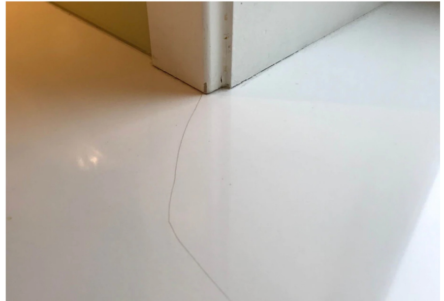
Quartz crack due to heat
